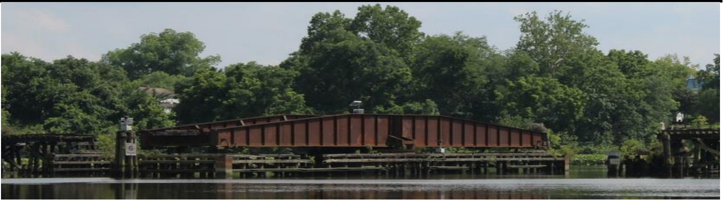
Current-day state of the Choptank River Railroad bridge. (Photo by Kennedy Thomason)
