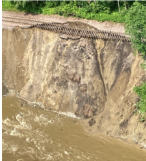
A slope failure on the Green Mountain Railroad at East Wallingford, Vt., is one of the areas where repairs continue as Vermont Rail System recovers from flooding earlier this month.
